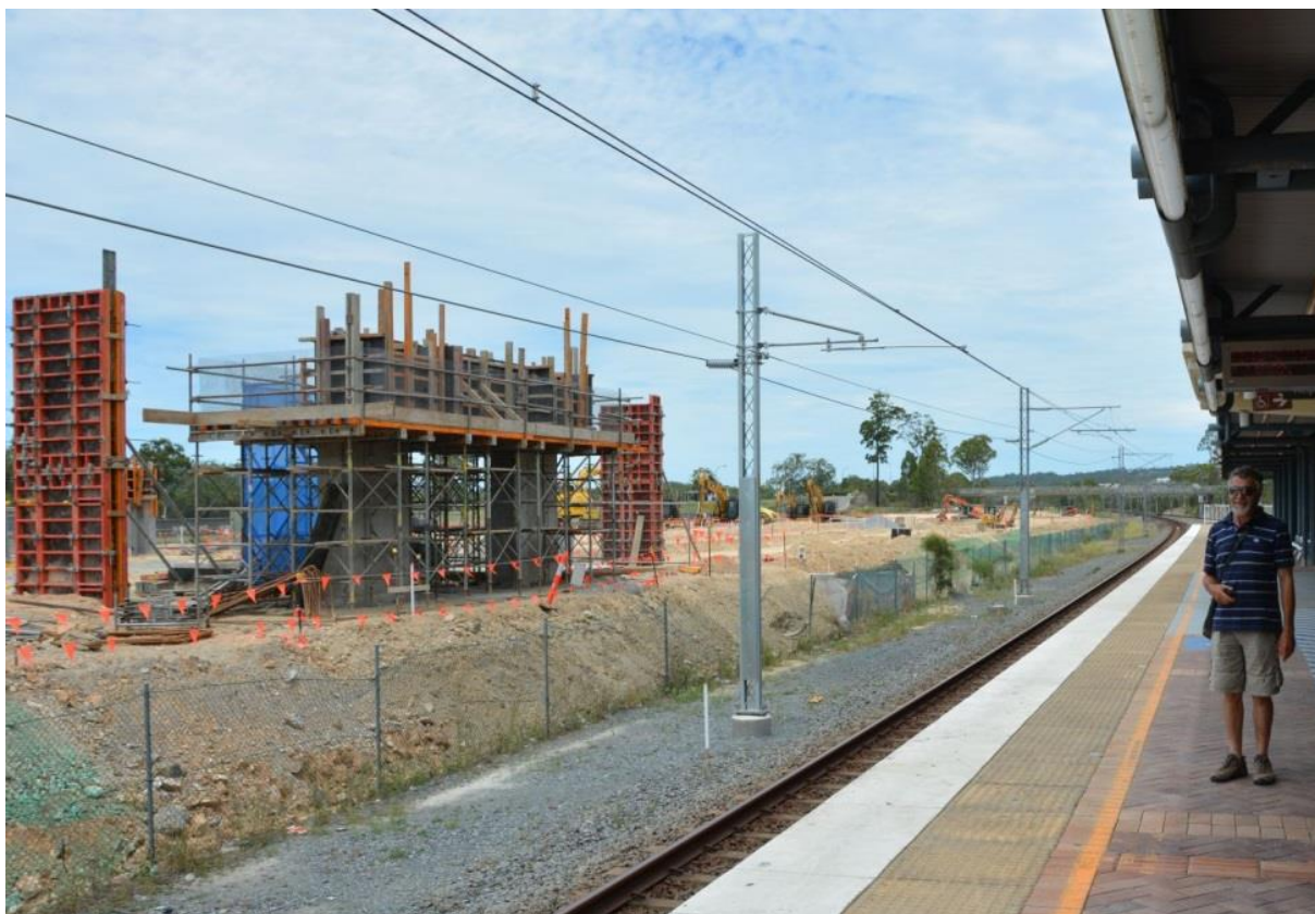
The Chairman at the site of the Helensvale tram-train interchange under construction (Mal Rowe)
